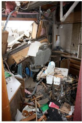
A close up look at what the tornado did to one of Dr. McGinty's treatment rooms. Photo by Craig Palmer
