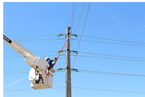
Photo courtesy of: the American Public Power Association
